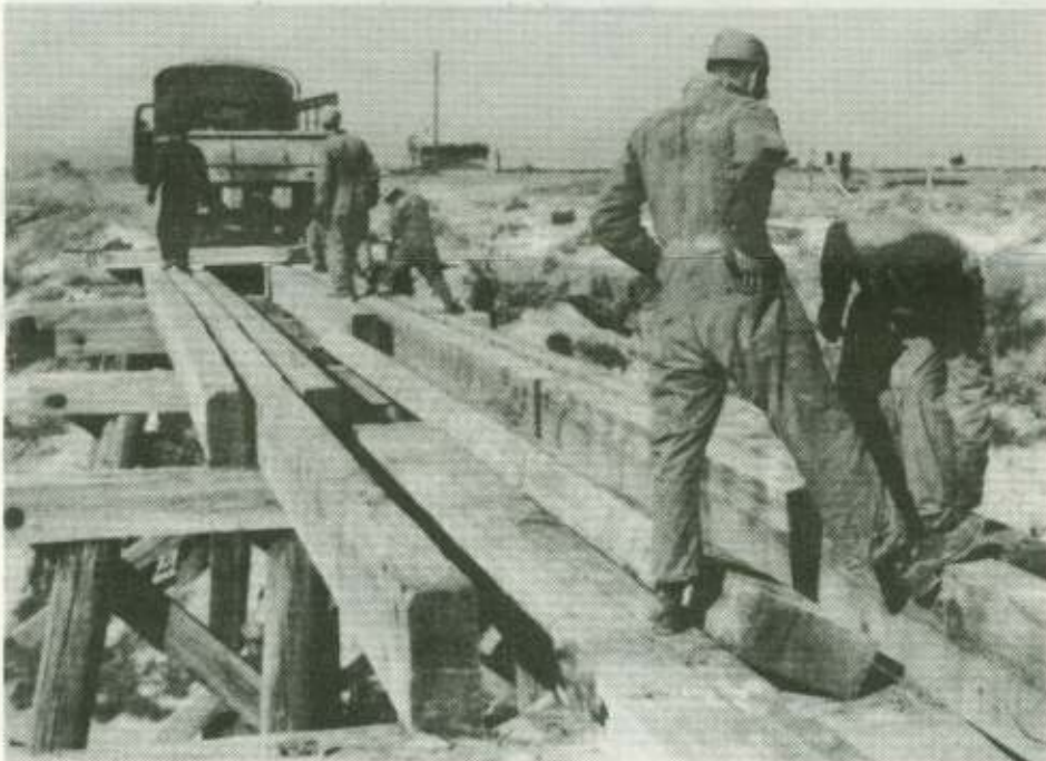
Removing an old railroad bridge at Gold Hill, Nevada, to salvage the timbers.
